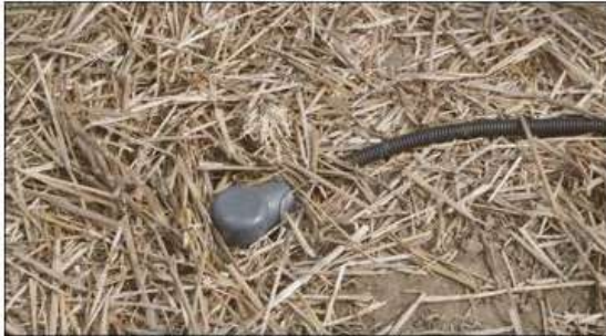
Picture 27: After pouring the slurry mixture into the bored hole you can insert the probe. Probe should be inserted until only the top cap is visible above the surface.
